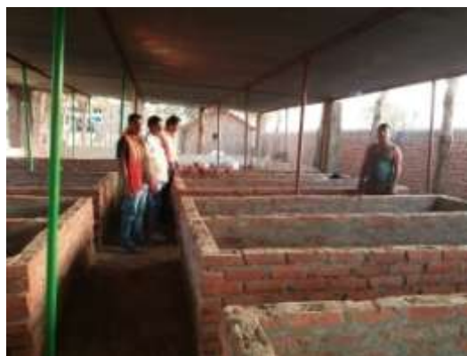
Long View of Unit
